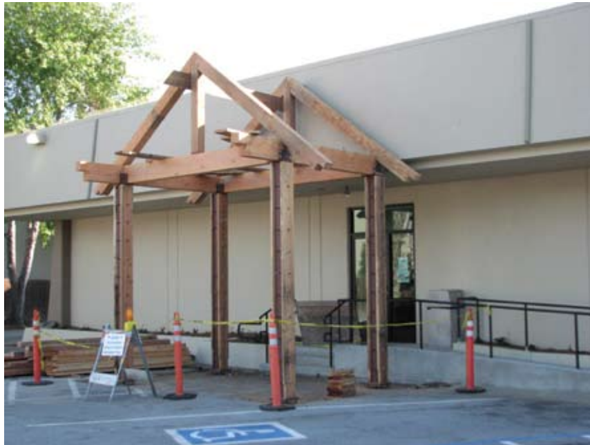
Our new gateway at the Foster City Service Center is coming along!
